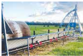
Above: H25MAX installed on a centre pivot in Marcollat, SA - 2022
